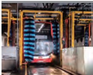
With the environmental-friendly design, the automatic waste water treatment systems properly treat effluents
