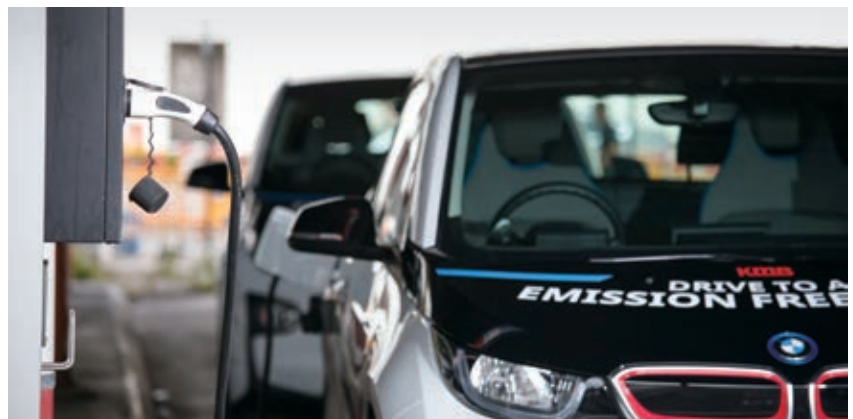
○ KMB and LWB have installed electric patrol car recharging facilities in their main depots
